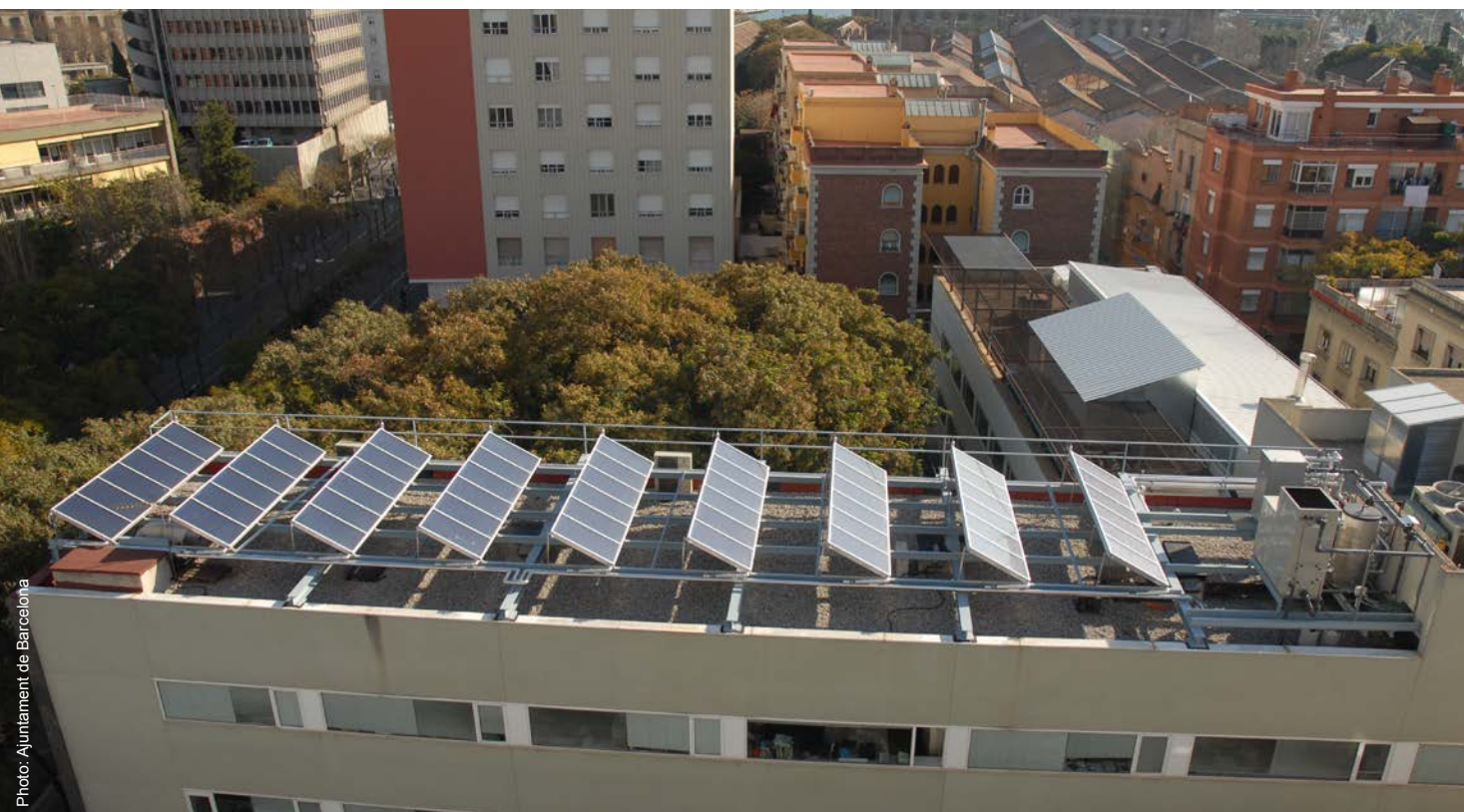
Local government leading the way: a solar energy installation at the Public Health Agency Laboratory
