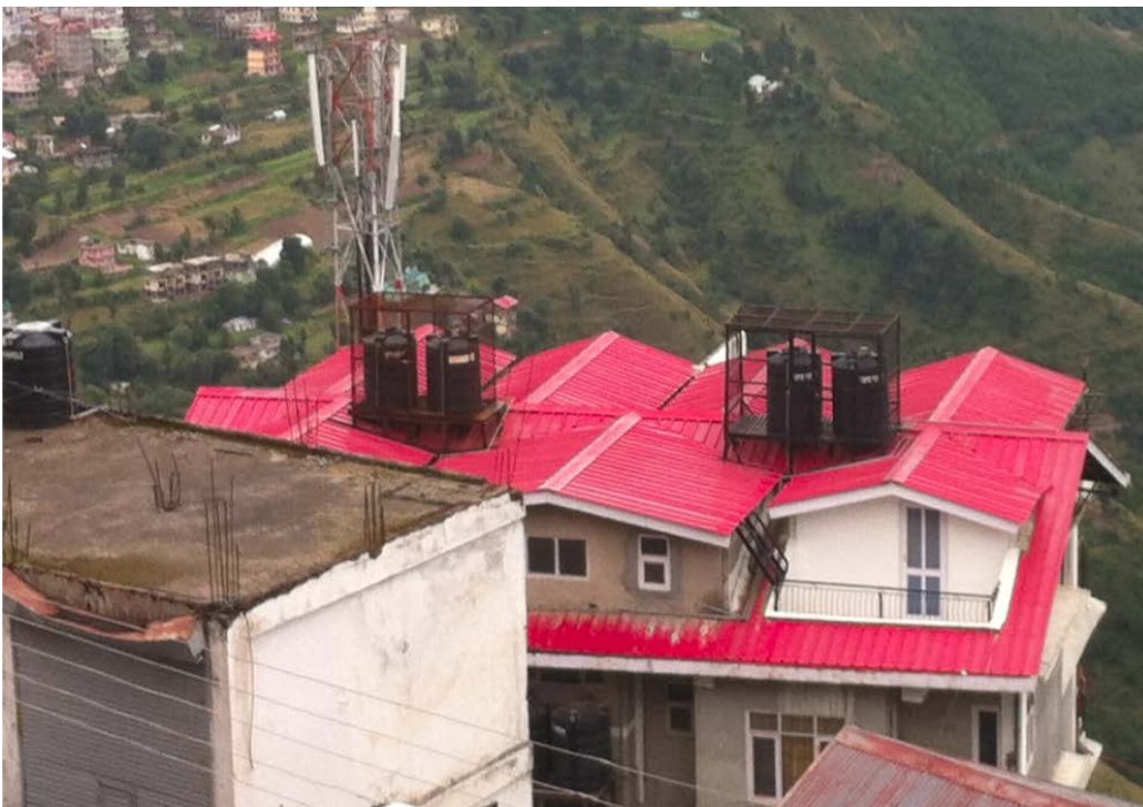
Figure 4: Installed rainwater tanks for harvesting © ICLEI
