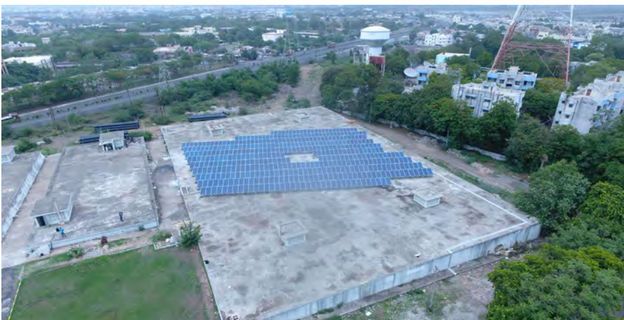
Rajkot, India, Urban-LEDS project city, has installed a 145kWp solar PV system to help power its Aji water treatment plant
