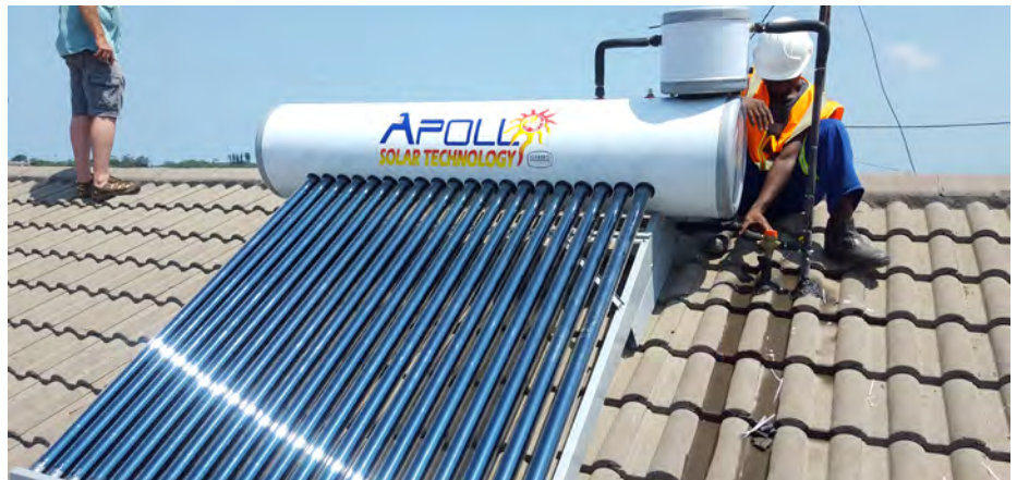
Solar water heaters save electricity and money – here installed on Groutville Care Homes in KwaDukuza, South Africa, as a pilot project implemented by Urban-LEDS in phase 1
